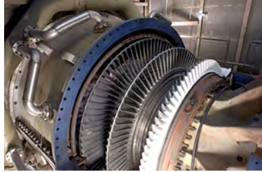
Figure 20.29 Steam turbine generator. The steam produced by burning coal impacts the turbine blades, turning the shaft which is connected to the generator. (credit: Nabonaco, Wikimedia Commons)
